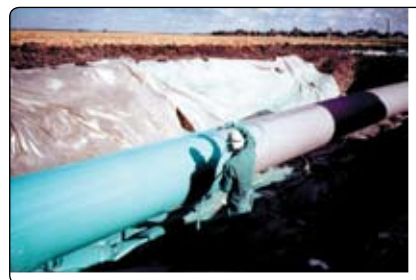
3M™ Scotchkote™ liquid epoxy being applied to a pipe for a rehabilitation project. 21
