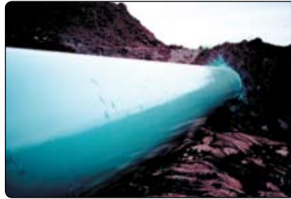
Pipe rehabilitation project completed using 3M Scotchkote coating — and repaired with Scotchkote hotmelt patchsticks. 6
